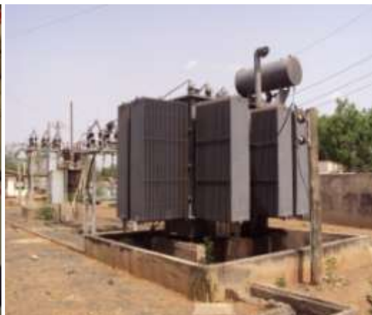
Plate 5.6: injection sub-station switch yard [26]
