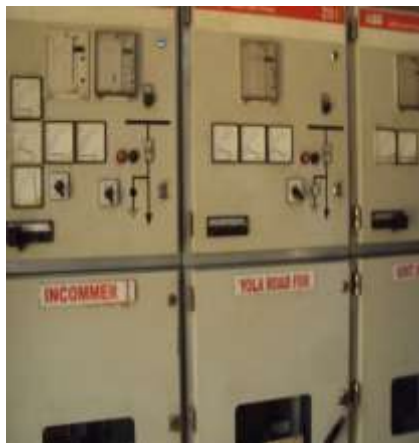
Plate 5.5: 33KV Metering Point [26]
