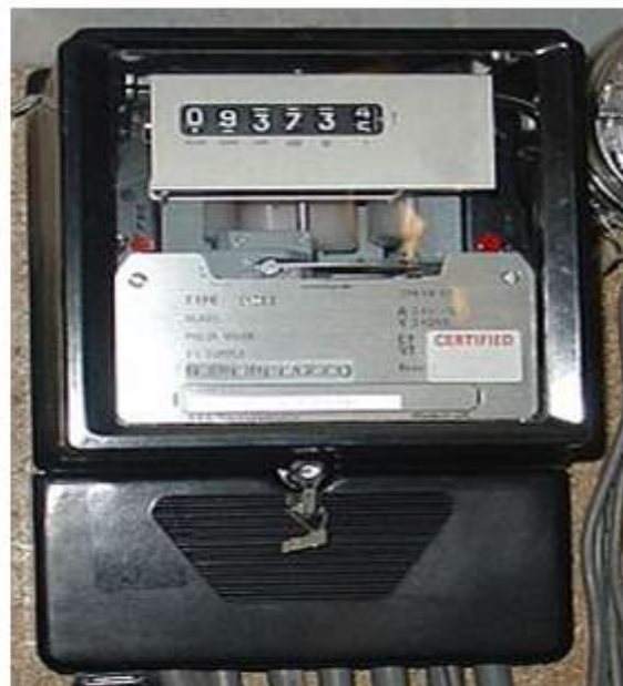
Plate 5.2: Electromechanical Energy Meter [26]
